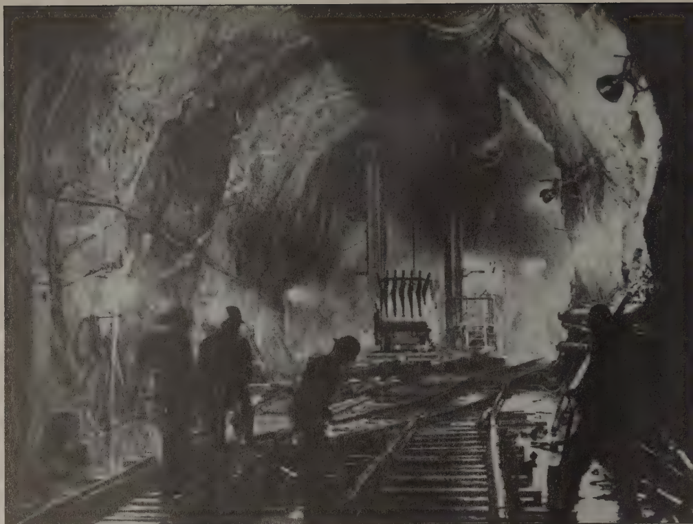
A large water distribution tunnel being carved through rock 700 feet below Manhattan. In some places, city water tunnels such as this reach 2500 feet below the surface.
